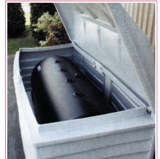
Many homeowners now have aboveground tanks installed inside tank enclosures, such as the one pictured here.
